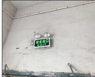
Photo of fire safety equipment 2 Exit sign and Emergency light.jpeg
