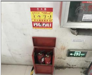
Photo of fire safety equipment 2 Fire extinguishers.jpeg
