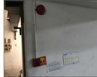
Photo of fire safety equipment 2 Fire alarm system.jpeg
