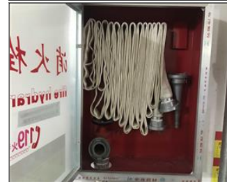
Photo of fire safety equipment 2 Fire hydrant.jpeg
